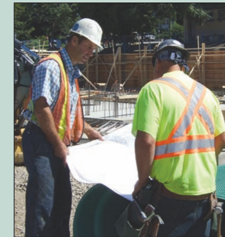
Contractor Chuck Winn (L) and Guy McLean (R) review blueprints for Nixon Wenger's new office building, under construction at the corner of 28th Street and 30th Avenue.
